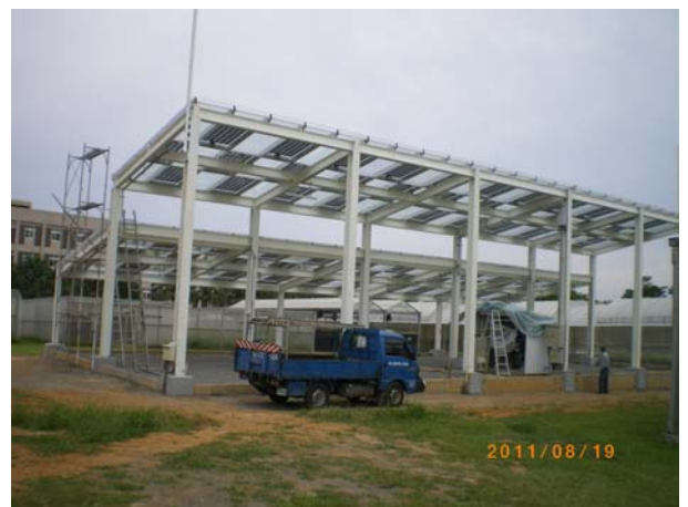
Solar energy production capacity in fruit and vegetable greenhouse area
